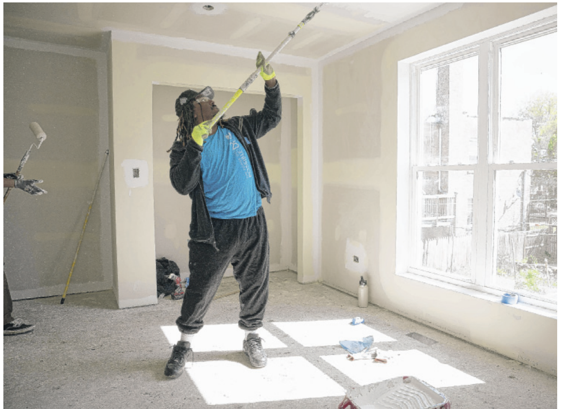
Volunteer Jonathan Festherson paints a house near North Lockwood Avenue and North Laramie Avenue in Austin on Saturday.
